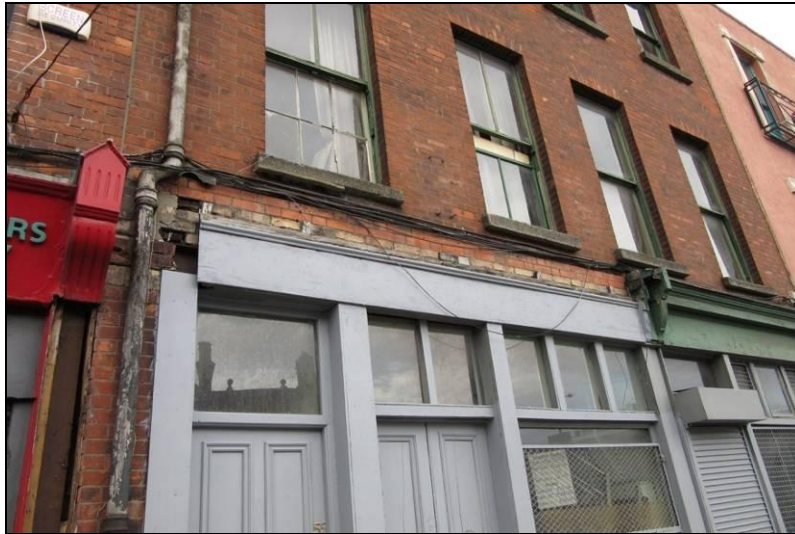
Figure 6: View of fascia of shopfront and missing cornice and console brackets
